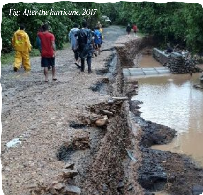
Fig: Erosion defence
